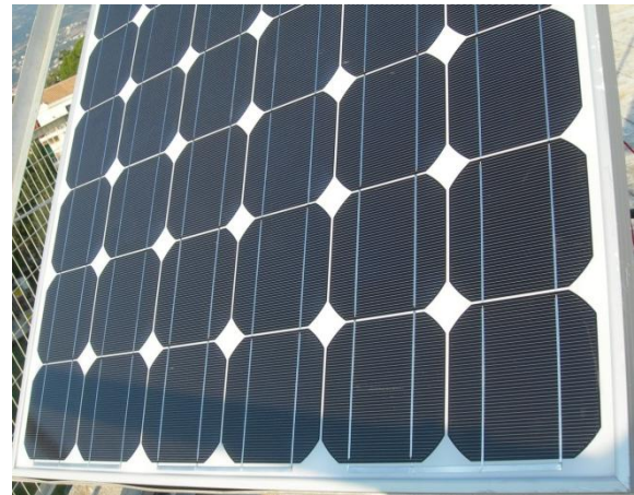
Fig. 4. PV panel partially shadowed by a pole. The thick line of the shadow in the bottom part of the panel crosses all the 6 strings, which are at vertical direction.
