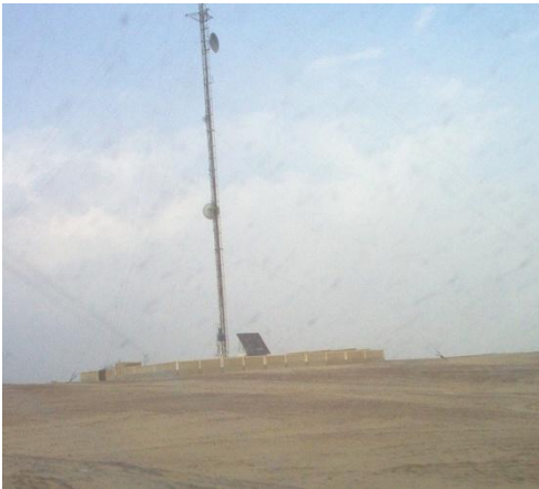
Fig. 7. SAPV system powering a telecommunications station in the middle of the desert outside Kairo, Egypt.
