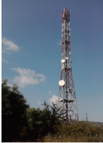
Fig. 1. A PV powered telecommunication system near Pyrgos, Greece.
