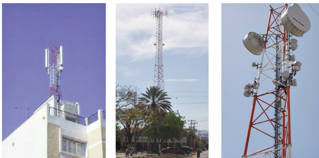
Figure 5. Several antenna types mounted
